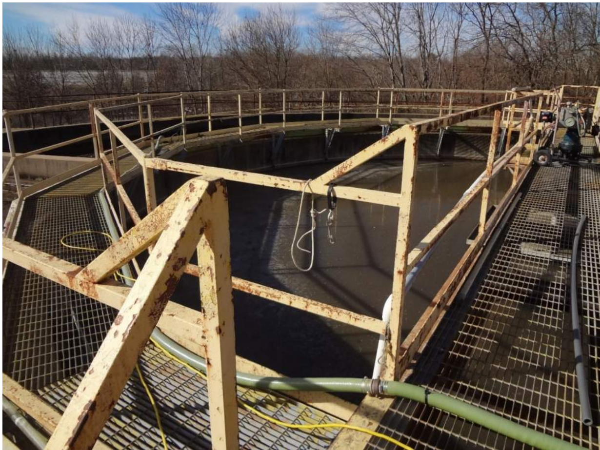
Figure 5-19: Solids Handling Tank and Walkway
