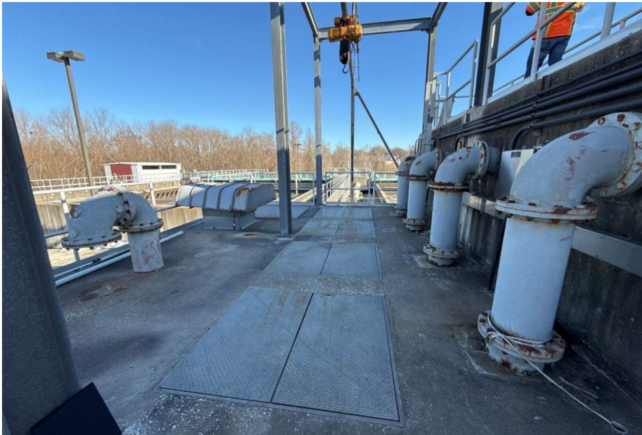
Figure 5-1: Influent Pump Station
